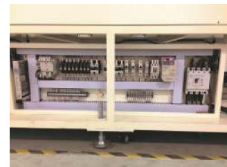
Power switch box for the control of curing oven
