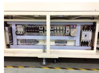
Power switch box for the control of curving oven
